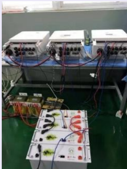
Multiple machines in parallel
